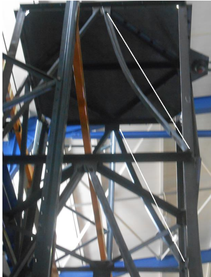
Figure 7.19: Tower O-1S. Weak axis flexural buckling of the failed diagonals towards the lips
