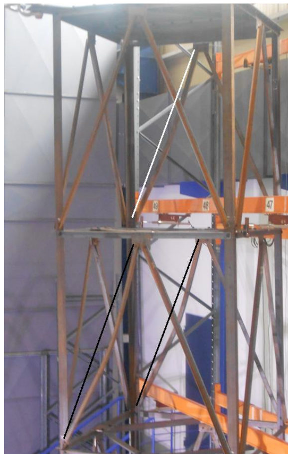
Figure 7.25: Tower D-1. Weak axis flexural buckling of the failed diagonals towards the lips
